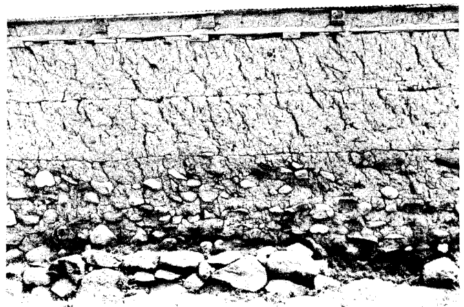
Fig. 51. Distinct layers of puddled clay are visible on this barn at the Grosz farm. Stones mixed with puddled clay occur regularly toward the foundation. Note the horizontal wall plate and shims embedded between the top tier of clay and the floor joists.
