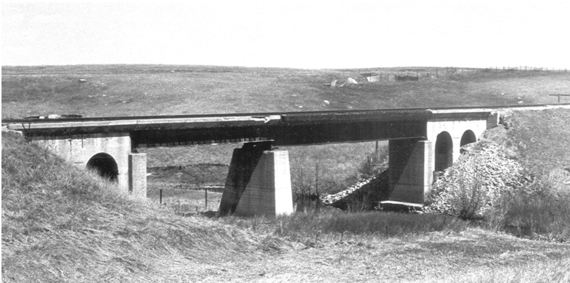
Figure 32. This deck girder bridge on the Milwaukee Road west of Aberdeen displays the arched concrete approaches that were characteristic of that railroad's larger bridges (State Historic Preservation Office photo).
