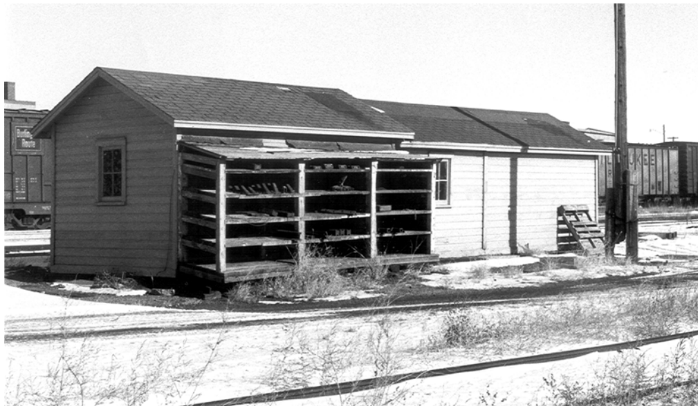
Figure 29. Tool sheds in the Milwaukee Road yards in Mitchell (State Historic Preservation Office photo).
